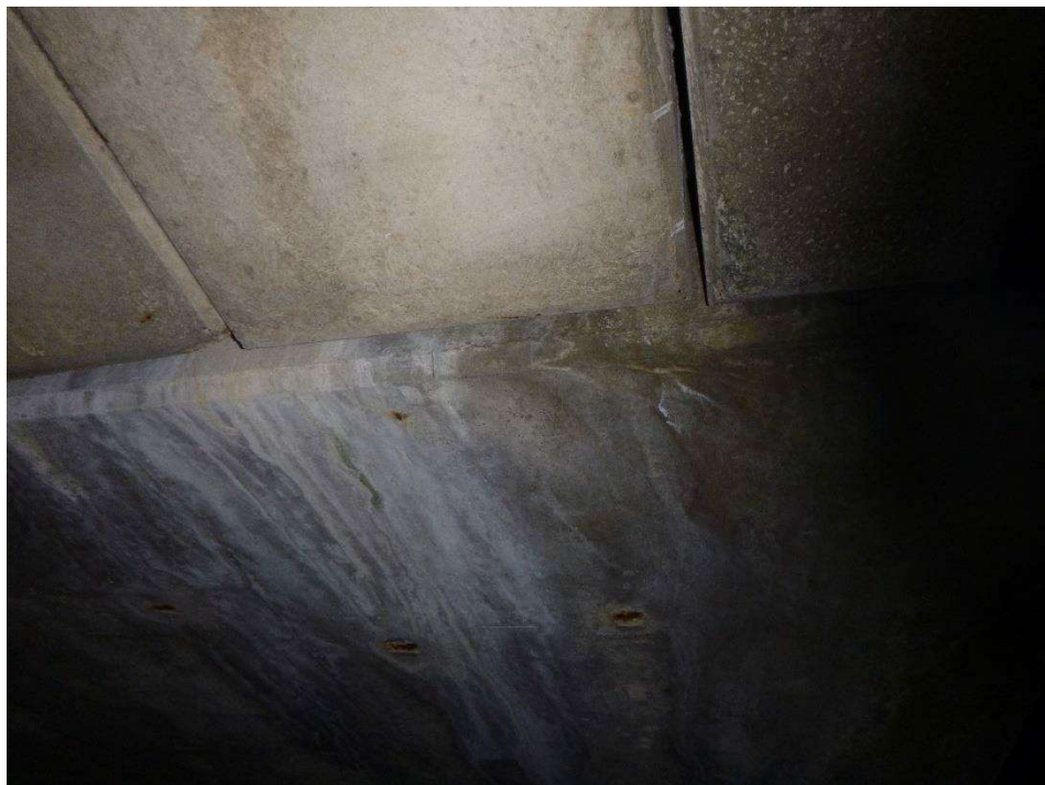
Photograph 10 - Leachate staining to deck soffit.
