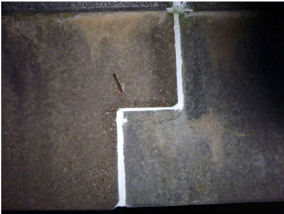
Photograph 2 – South-east half-joint. Note, previous repair and exposed reinforcement.
