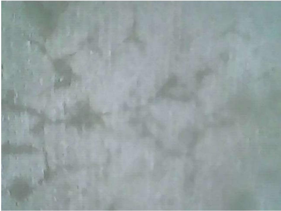
Photograph 5 - Shrinkage cracking to northern T-beam upper nib.
