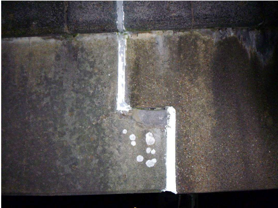
Photograph 3 – South-west half-joint. Note, previous repair and minor spalls.
