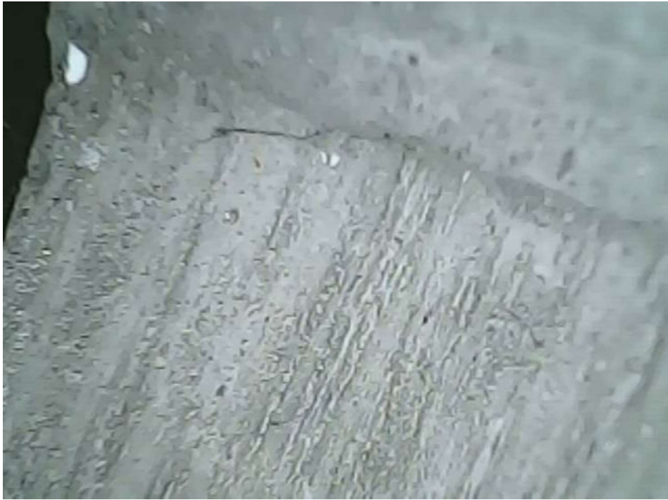
Photograph 9 - Crack to lower nib of south box beam.
