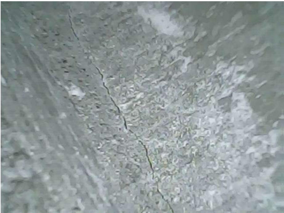
Photograph 8 - Crack to lower nib (2 nd beam from south)
