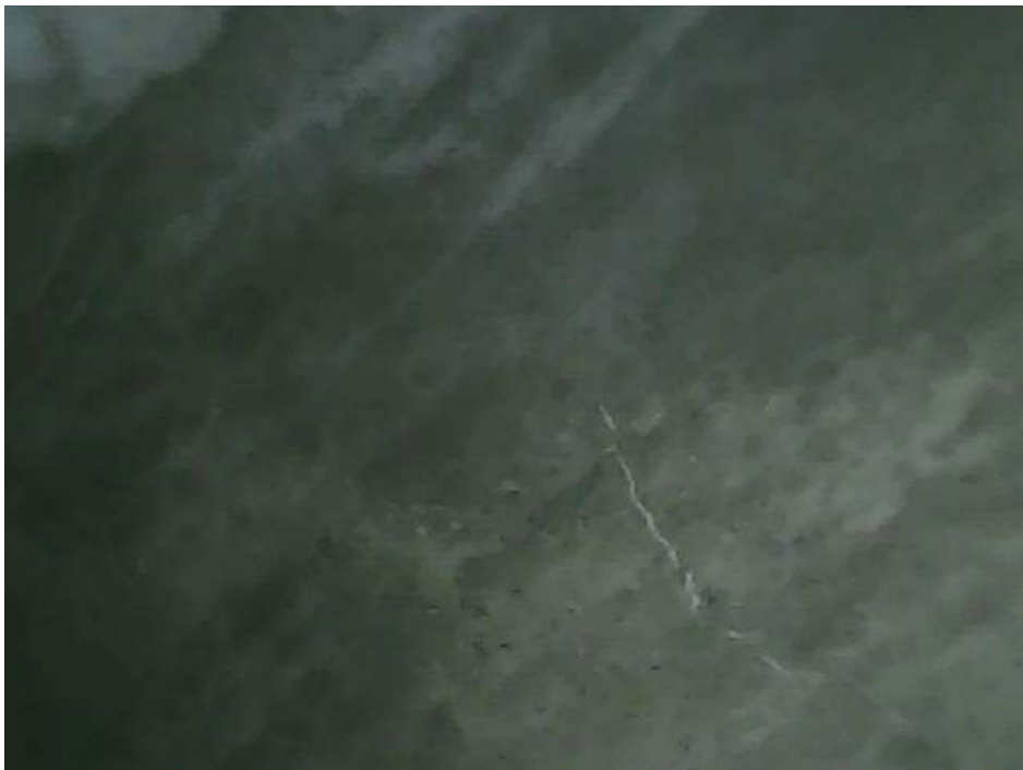
Photograph 6 - Crack to lower nib (north elevation)
