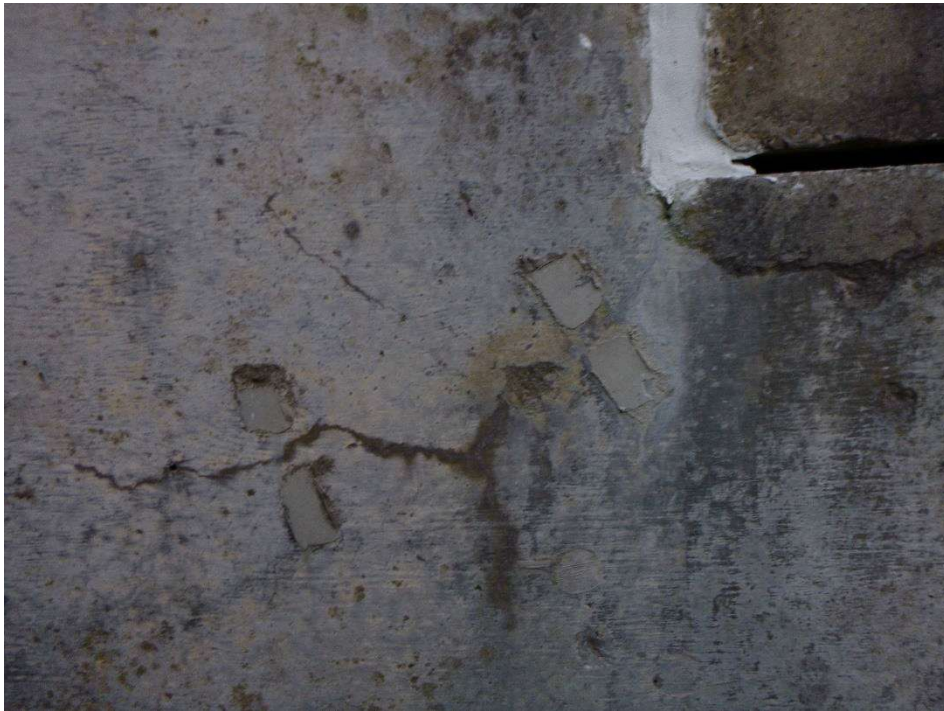
Photograph 1 - Close up on cracking to north-east half-joint
