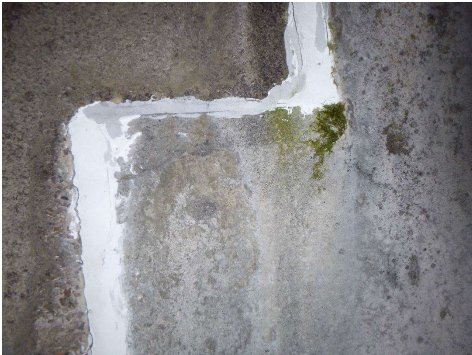
Photograph 4 - Algal staining and previous repair to north-west half-joint. Note, the joint is fully sealed.
