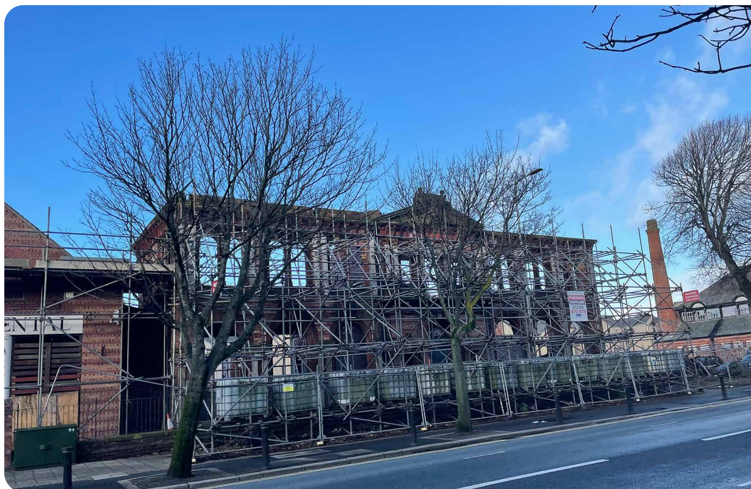
Fire damaged Grade II listed former Working Men's Club
